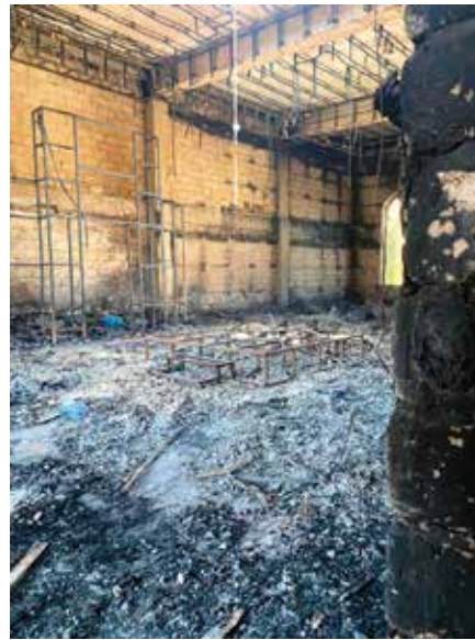
A burnt shul in Dagestan, Russia after terrorists set it afire.
